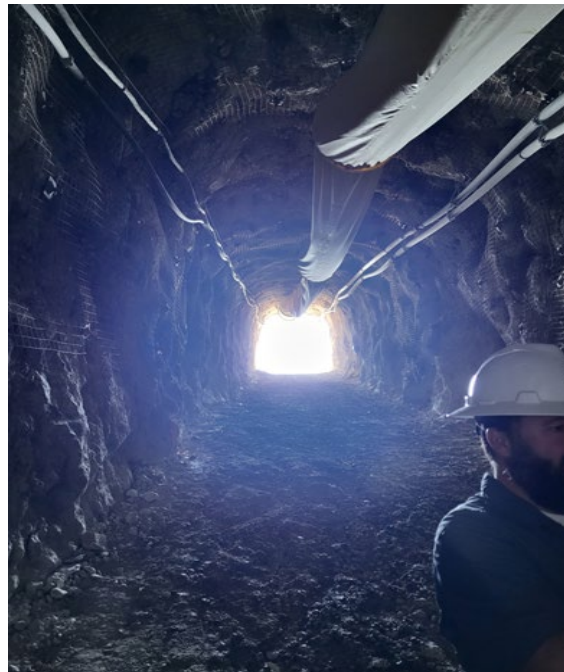
Decline and ventilation.
