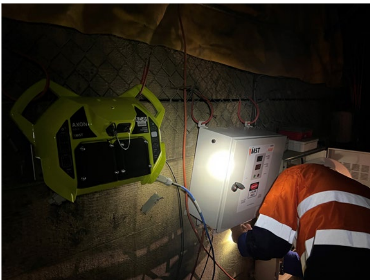
AXON Core, Composite Fiber Cable, and UPS AXON Mini installation
