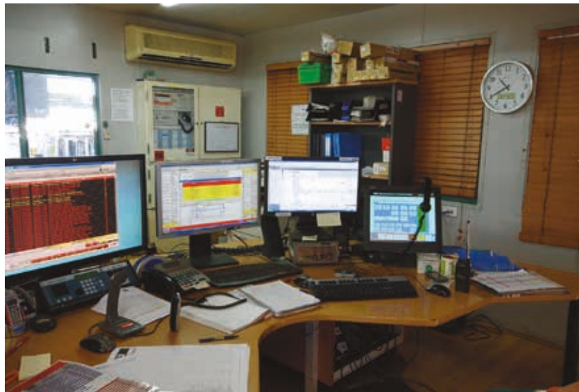
Information overload is a growing problem in the control room. MST’s integrated approach eliminates the need for multiple screens in order to view key information.
