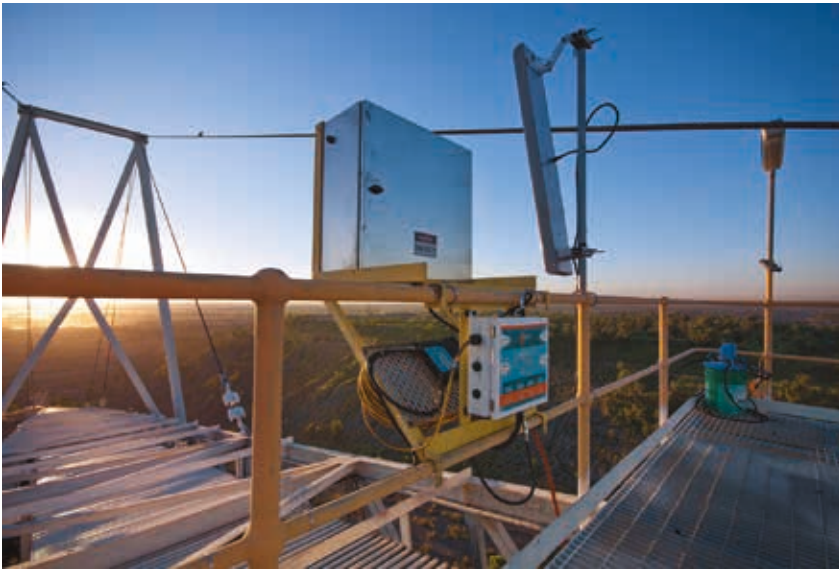
Mine Site Technologies (MST) provides a 360° coverage of mine operations with its ImPact Wi-Fi Digital network and integrated communications technologies.
